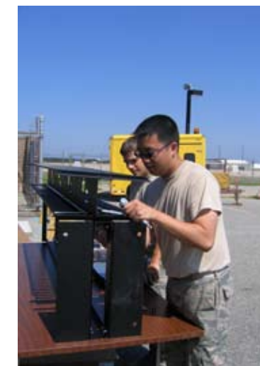
Senior Airman John Wong, 102nd ACOMS cyber transport systems journeyman, and Airman 1st Class Michael Servis, 102nd ACOMS cyber systems operations journeyman, assemble a cable rack used to support command and control (C2) equipment recently installed on Otis Air National Guard Base, Mass., as part of the 102nd Air Operations Group's new Air and Space Operations weapon system. The equipment installation was accomplished without interrupting on-going support of real world operations and supports the 102nd AOG's goal of attaining initial operational capability in April 2011.
